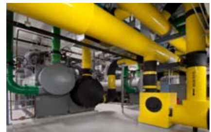
Nova Southeastern University, Central Plant
